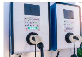
EV Charging, OBC, EVSEs
